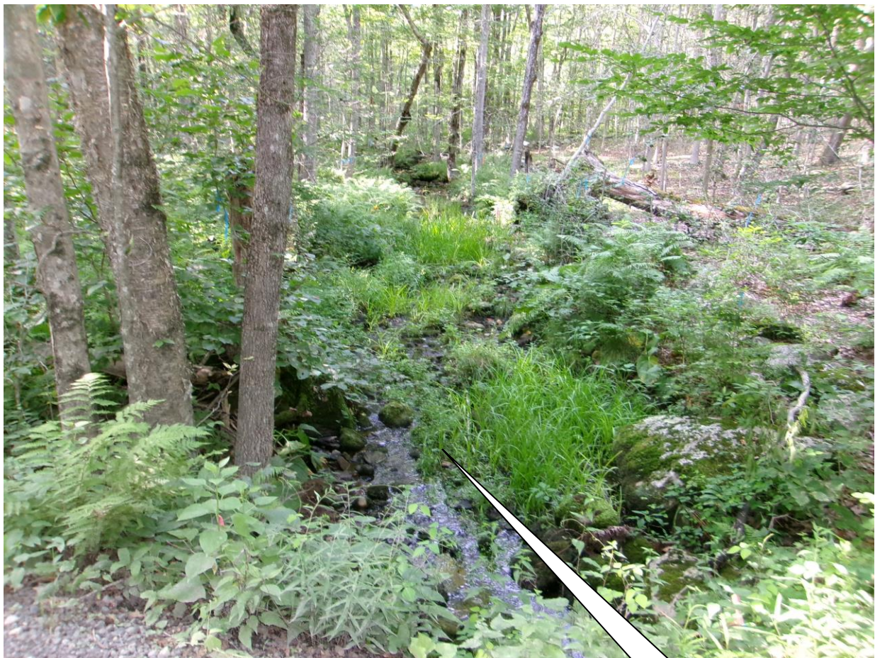
PICTURE NO. 2 LOOKING AT UPSTREAM (NORTH) OF EXISTING STONE CULVERT CROSSING OF ABNER LAND
